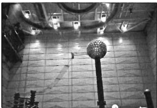
Impulse Generator inside the HV Lab
